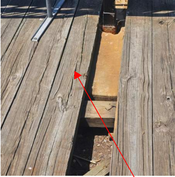
Generic decking showing splitting 8/21/2024
