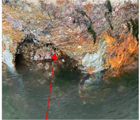
HOLE IN THE BACK OF PILE; PILE RANKED WITH ADVANCED DAMAGE
