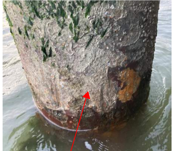
MINOR PITTING OF STEEL, SECTION LOSS AND RUSTING
