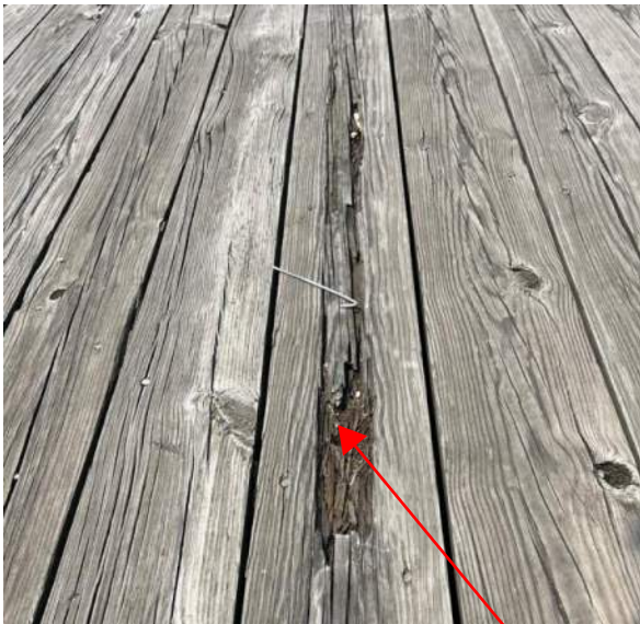
10-15% of decking requires repair or replacement 8/21/2024
