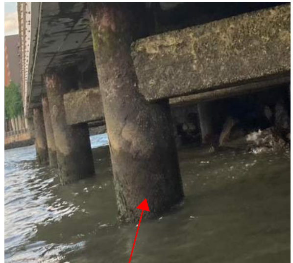
MINOR PITTING OF STEEL, SECTION LOSS
