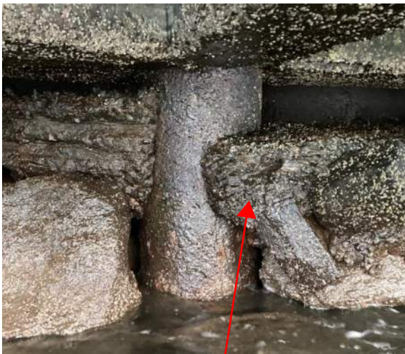
POTENTIAL DAMAGE TO PILE DUE TO DEBRIS. CONDITION. DAMAGE RANKED AS ADVANCED
