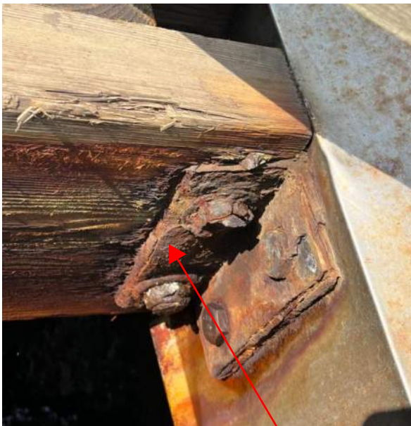
WOOD8 Rusted hardware 8/21/2024
