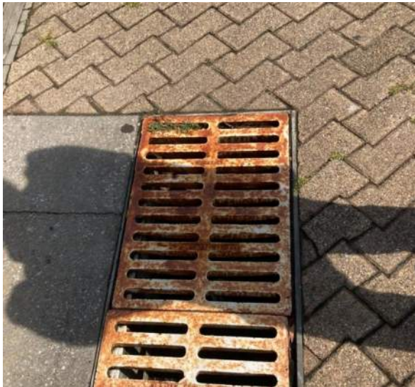
Minor Rust in Drain Covers 8/21/2024
