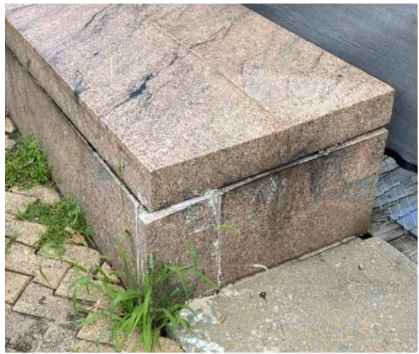
Stone displacement; loss of grout at joints 8/21/2024
