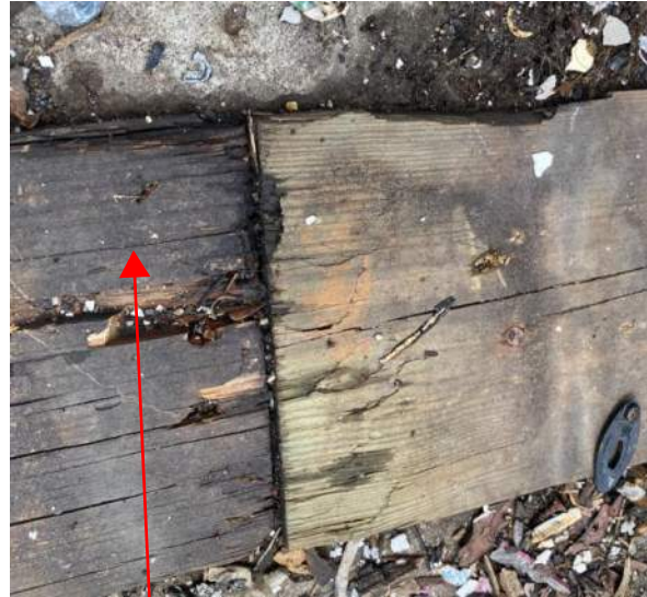
Embedded nailers show sign of rot 8/21/2024
