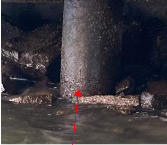
MINOR PITTING OF STEEL
