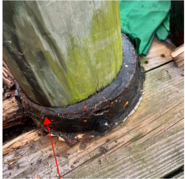
RUSTING ON BASE OF LIGHT STANDARDS
