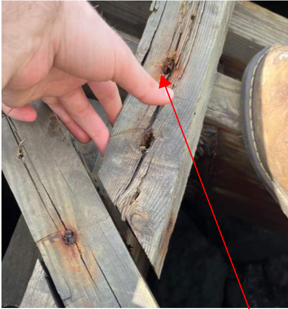
WOOD6 Split framing at rusted hardware 8/21/2024
