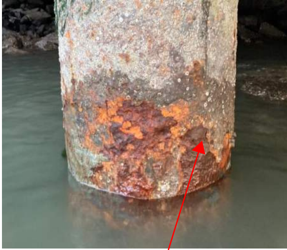
MAJOR PITTING OF STEEL, SECTION LOSS AND RUSTING; PILE RANKED WITH ADVANCED DAMAGE
