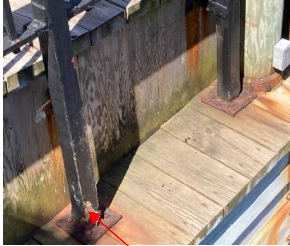
DAMAGED DECK POSTS
