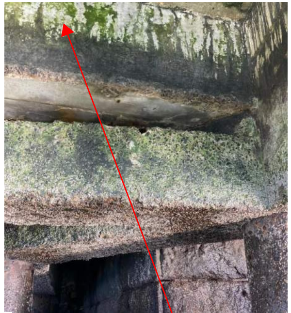
CONC9 UNDERDECK 8/21/2024 BIOLOGICAL GROWTH, SCALING
