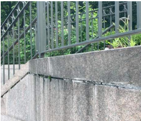
Loss of mortar at joints 8/21/2024
