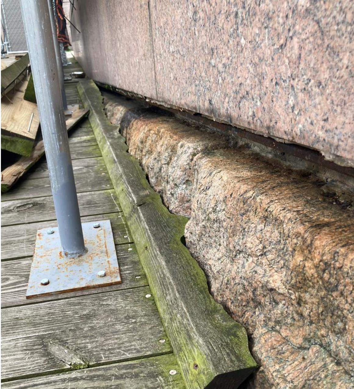
Rusted relieving angle at stone Joint has been caulked creating trapped moisture 8/21/2024
